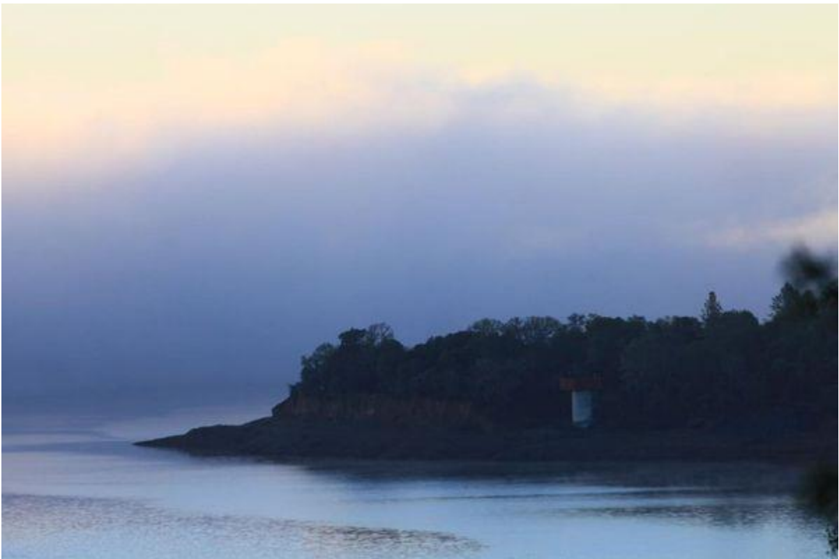
RVCWD pump house and intake at Lake Mendocino, by CJ Watt
