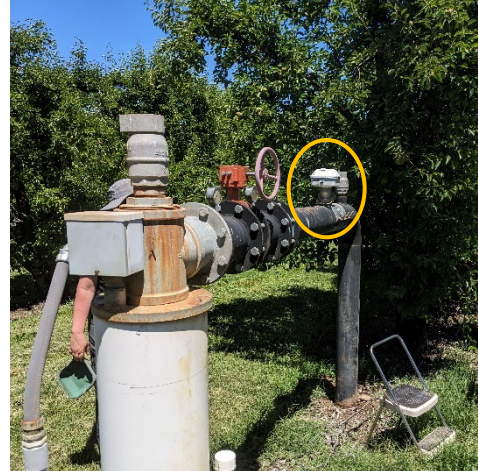
Figure 3. Pipeline for underflow well. An in-line water sensor and data logger are circled in orange.
